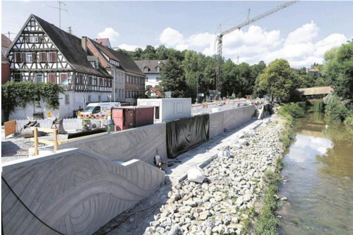
Fig. 2: Construction of Flood Walls on the Talstrasse in Backnang (Source: Photo by the author)
